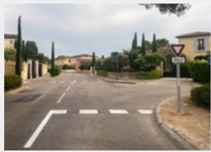
Installation of a give way on Chemin du Moulin de Vernègues, at the crossing of Rue de la Cascade.
