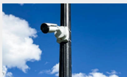
Installation of cameras for the Domain's video protection system.
